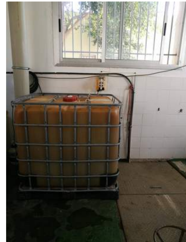
Anox Systems EBAR B
